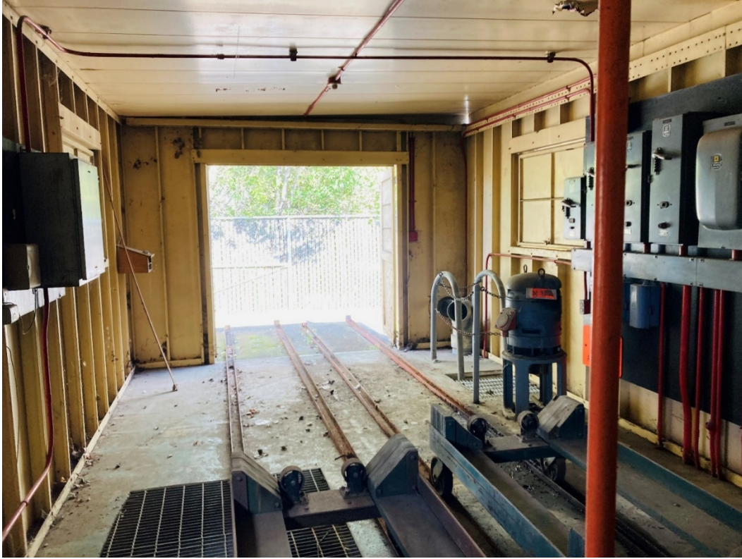
Interior of the chlorination structure, view towards the door, subfloor level entrance on the left of the door
